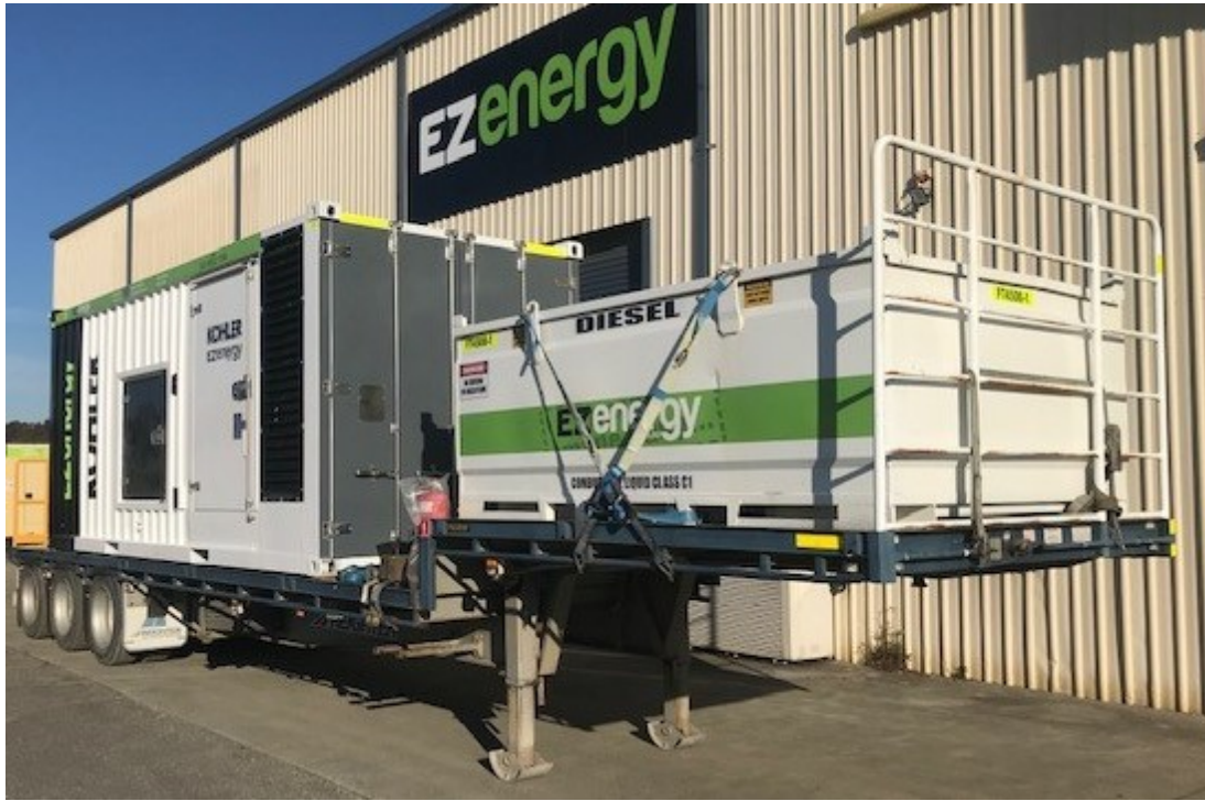
Emergency & Standby power ready to go
